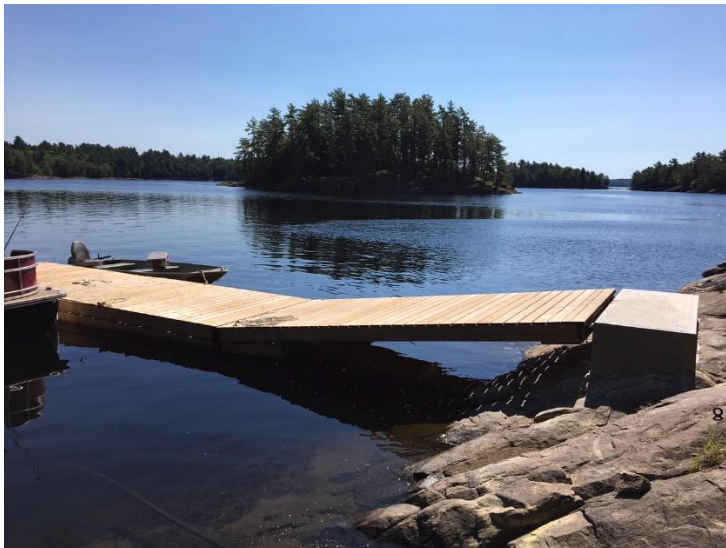
Late June installation of new bulkheads for dock by Ed Bennett and photos of the dock installed.
