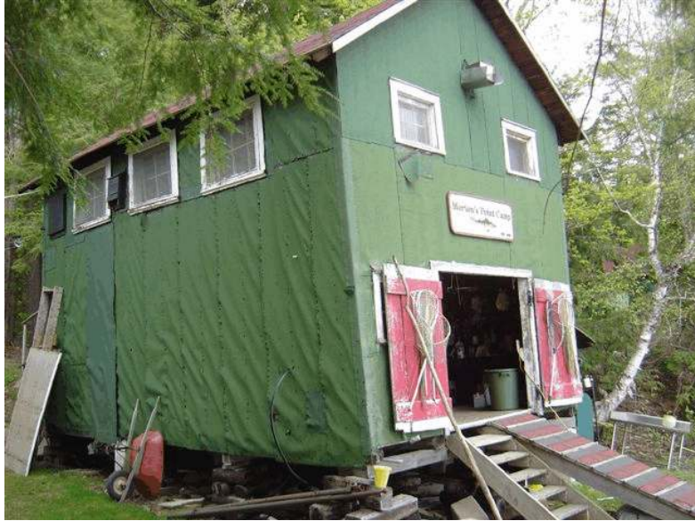
Crib work in poor condition May 2005.
