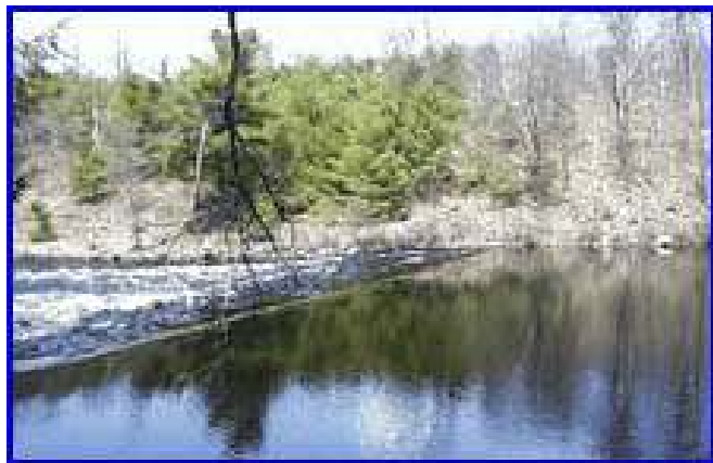
Dam on the Magnetawan River below Camp. May 2002. Work completed in September 2002.
