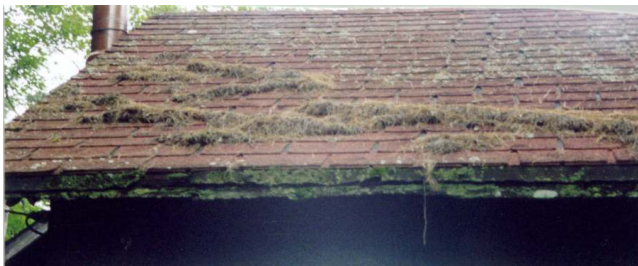
Cook's Cabin roof and fascia in need of repair. Picture taken August 2000 by Keith Balfour.
