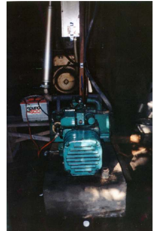
Front Onan generator. Rear Kohler generator
