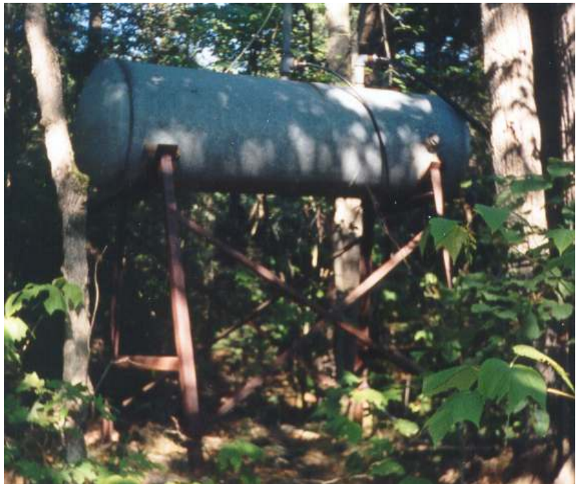
Water holding tank. Picture taken in August 1999.
